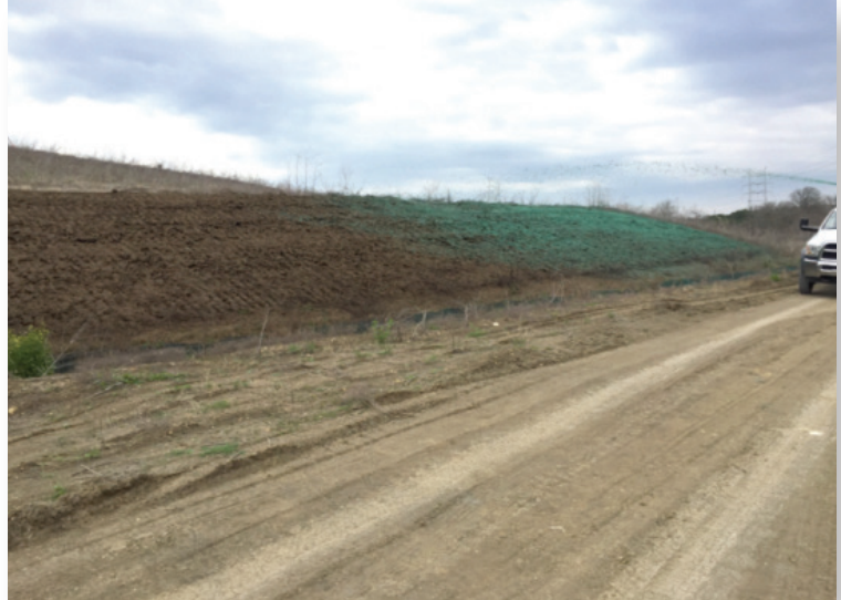
Installation of biotic Earth March 2018, covered with an FGM within the hour.
